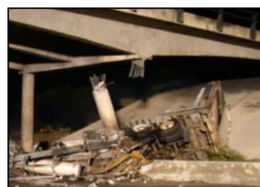
Figure 3: Impact damage of a bridge column
